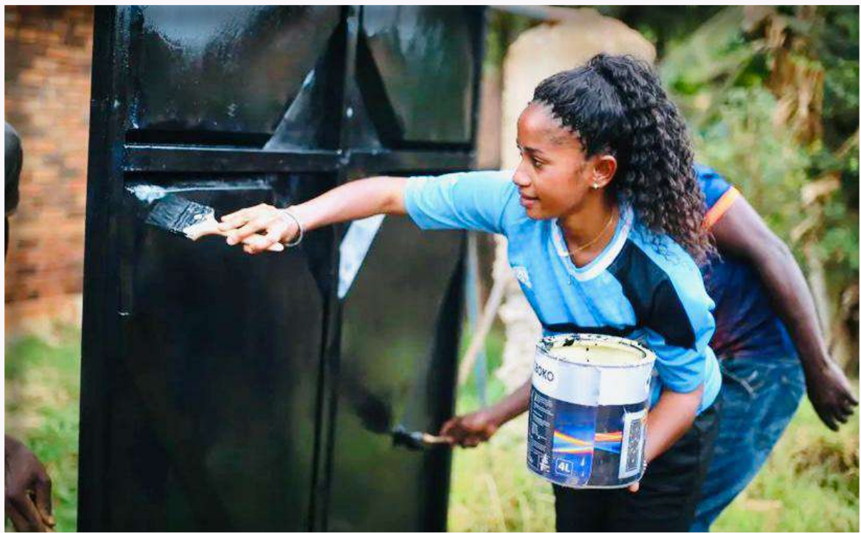
Foundation volunteer Natasha Mwaibula renovating by painting an entrance gate of Mehayo orphan center in Morogoro.
